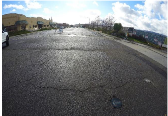
Intersection at Pasadena St. and Crane St. Photo taken on February 23, 2022, facing southeast.
