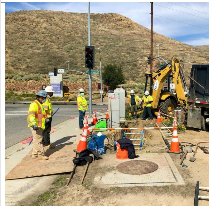
Figure 7. Undergrounding activities at the intersection of Indian Truck Trail and Temescal Canyon Road, March 17, 2021
