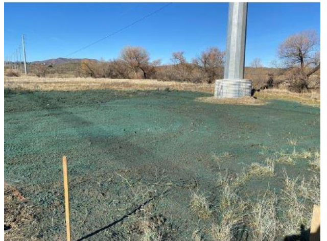
Feature ID: San Jacinto River. View of work area that was hydroseeded at Pole 4765121E post-construction. Photo taken on January 5, 2022, facing northwest.
